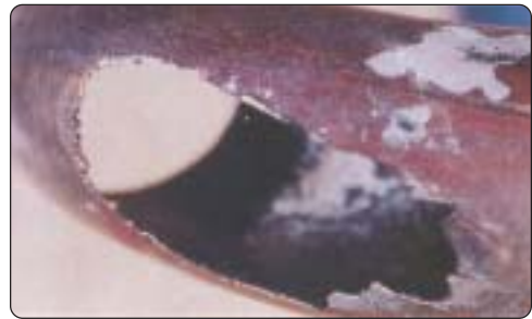
Fig. 1. Metal Erosion in U-bend.
